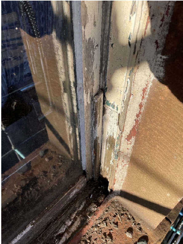
W5. Significant decay evident. Partial loss of cill and parting bead and glazing putty. Evidence of previous scarf repairs.
