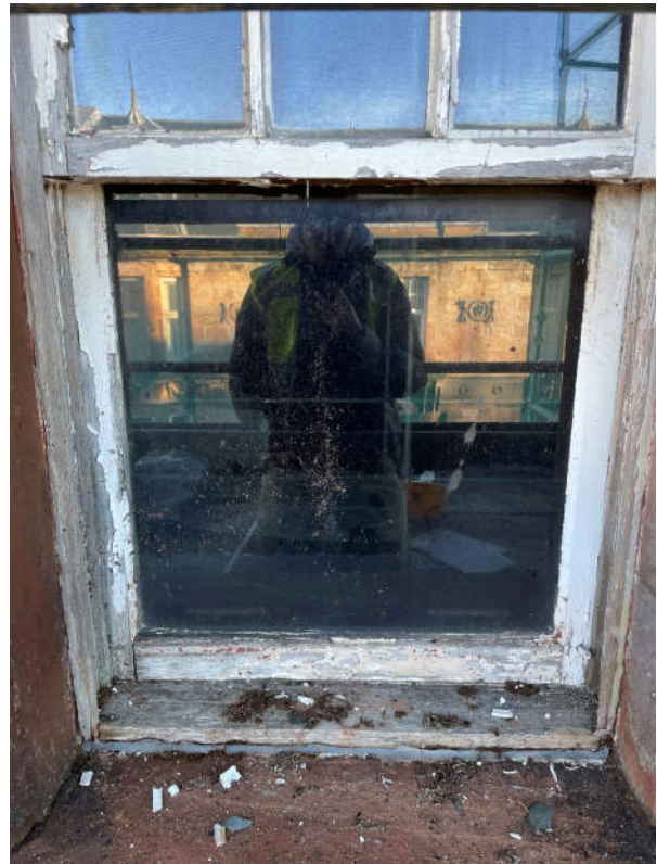
Window 'W3'. Lower sash in similar condition with loss of finishes. The timber was soft to the touch and became friable under pressure.
