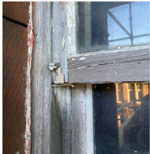
W4. Window in poor condition with splits in the meeting rail, lost fixings, and soft timber due to failed paint coatings.
