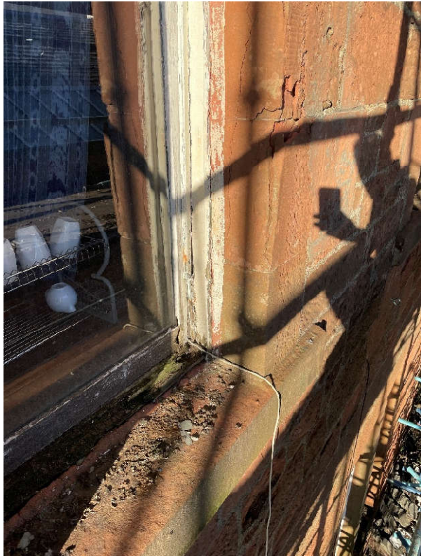
W8. Significant decay evident to bottom rail, sash slide and cill beyond repair.
