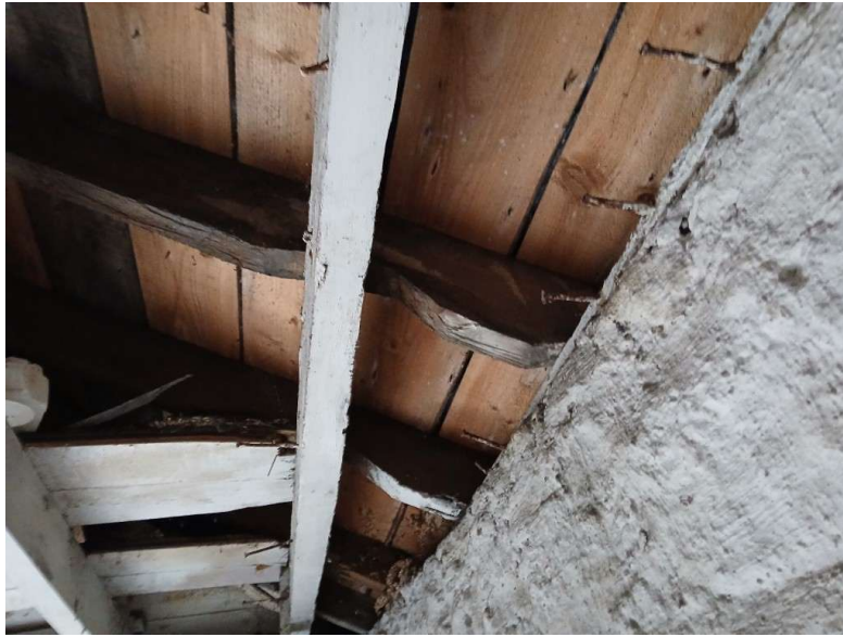
Photograph No.33 – Condition of timber elements various throughout the roof structure.
