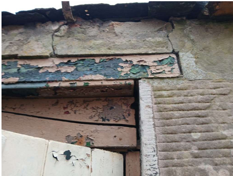
Photograph No.12 – Split in timber to lower lintol above door, flaking paint to upper lintol, opening up of joints in stonework above lintol.
