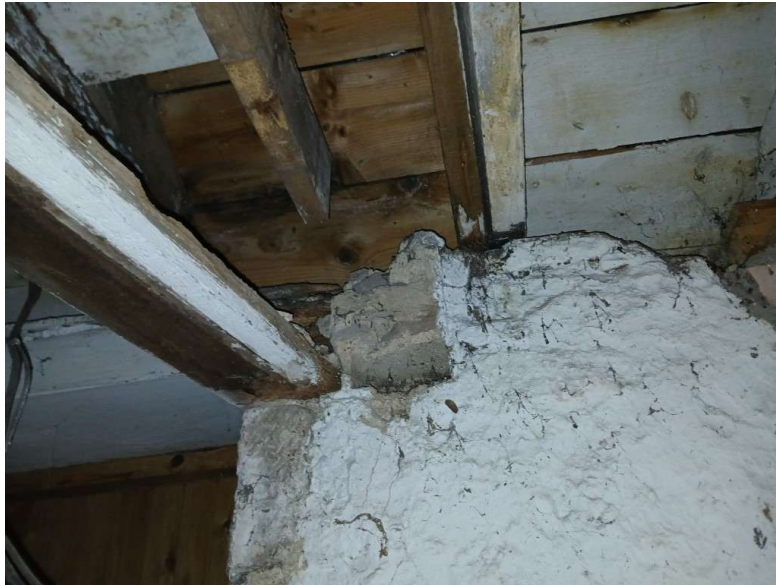
Photograph No.27 – Unsupported ceiling joist.
