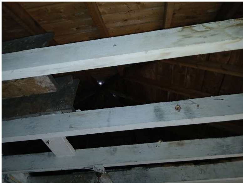
Photograph No.34 – Light visible indicating at least one hole in roof slope.
