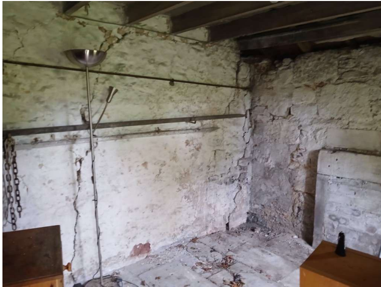
Photograph No.17 – Interior of southern portion of building viewing dividing wall running east-west. Extensive cracking visible and sloping of flagstone floor towards eastern gable.
