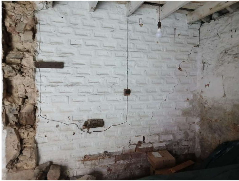
Photograph No.29 – West end of internal wall. Constructed with bricks on their side, step cracking in walling.
