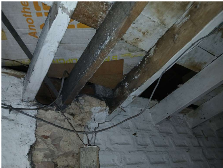
Photograph No.30 – Unsupported joist end at former dividing wall location.
