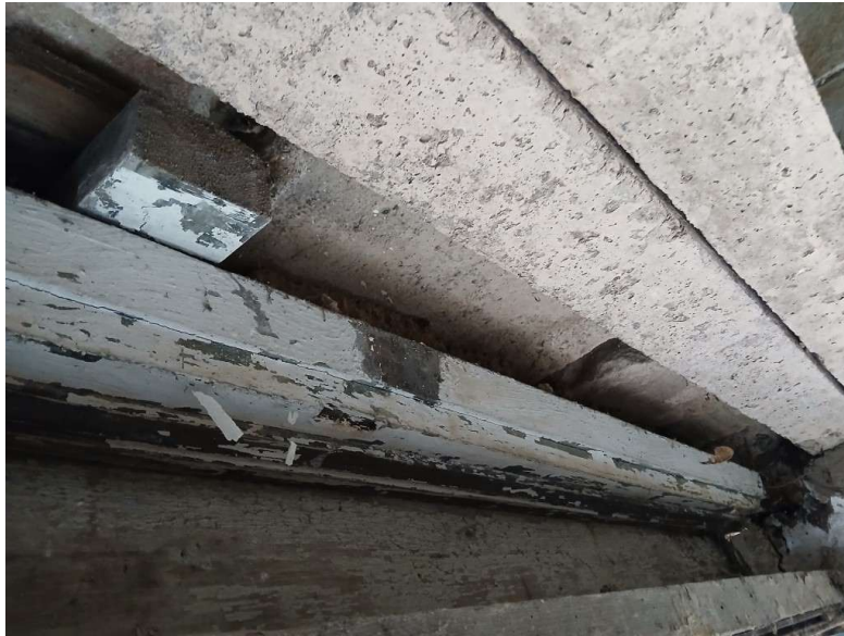
Photograph No.25 – Stone to outer leaf partially supported on external timber lintol and internal precast concrete lintol.
