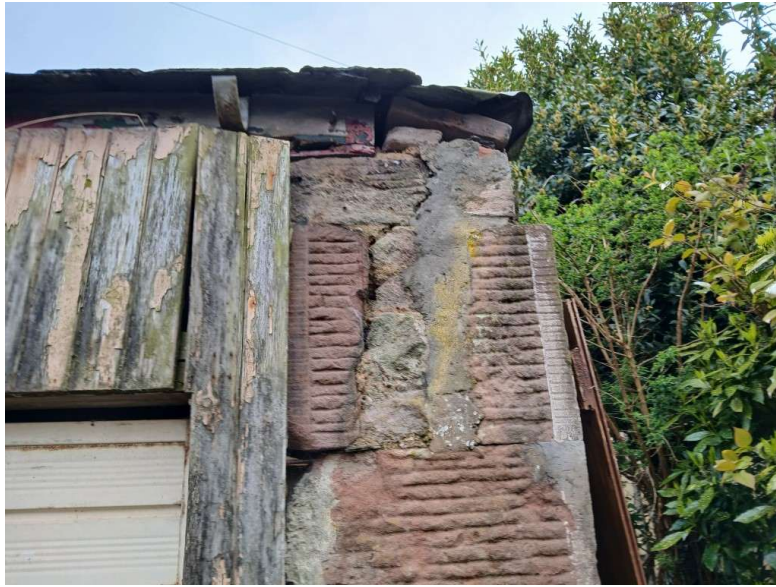
Photograph No.13 – Opening up of joints in masonry to north-western corner of building and timbers above door in poor condition.
