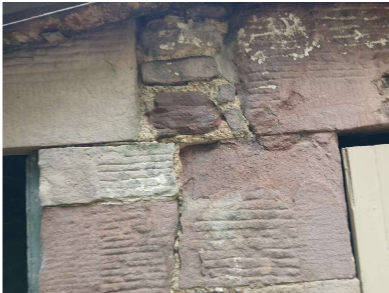
Photograph No.4 – Weathering and deterioration of stonework between doors on west elevation.
