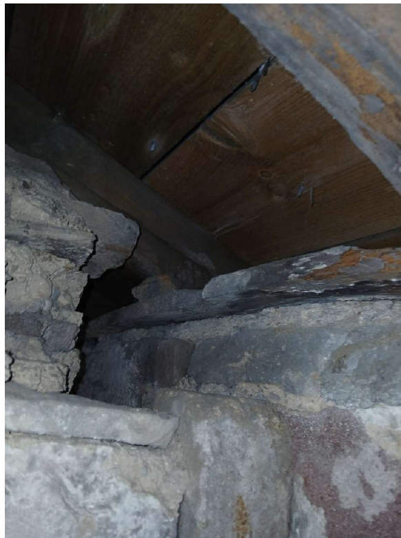
Photograph No.18 – Deterioration of timber and sign of woodworm visible on eastern gable
