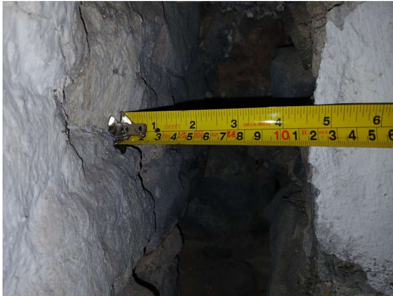
Photograph No.21 – 110mm gap at opening up/crack as photo 19.
