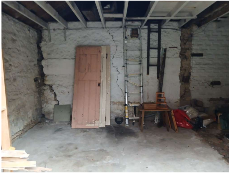
Photograph No.19 – Northern face of internal wall at eastern end. Large crack at intersection of eastern gable.
