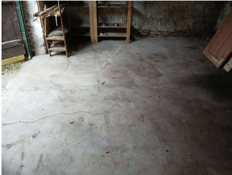
Photograph No.23 – Cracking noted across full extent of concrete floor slab.
