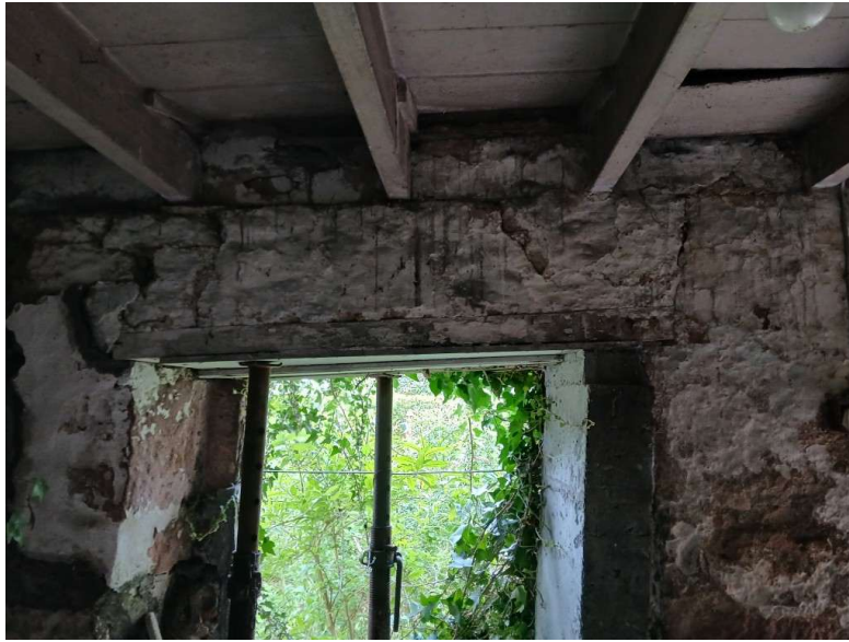
Photograph No.15 – Southern wall, internal. Window lintol propped in two places.
