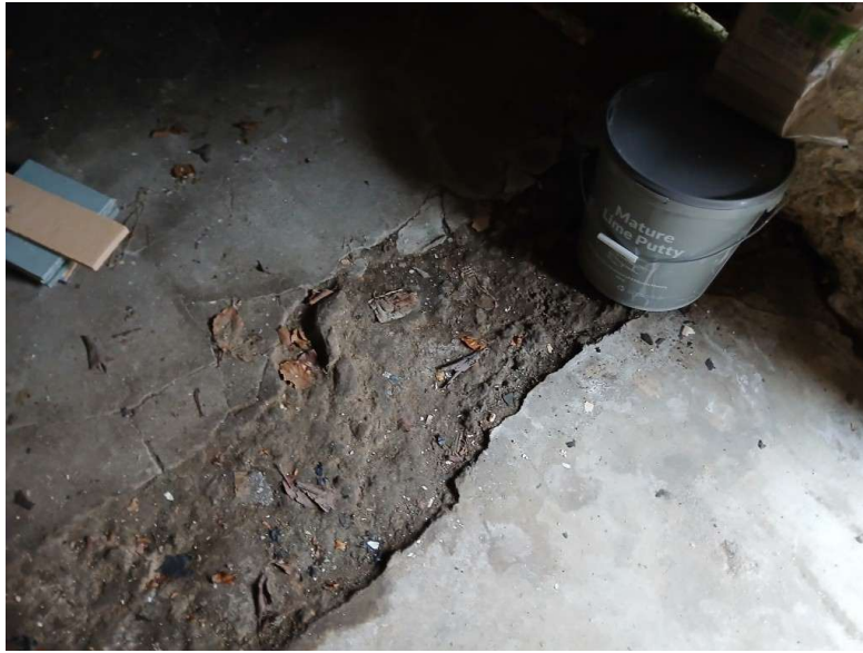
Photograph No.31 – No infill provided to flooring at former dividing wall.
