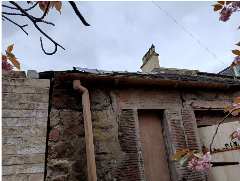
Photograph No.10 – Cracking to each side of window lintol and opening of joints.
