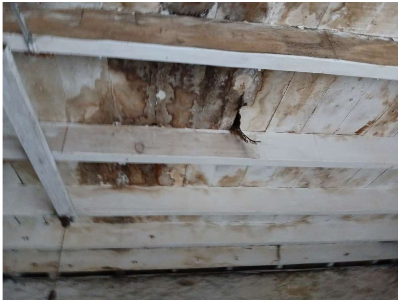
Photograph No.32 – Timber elements in .poor condition.
