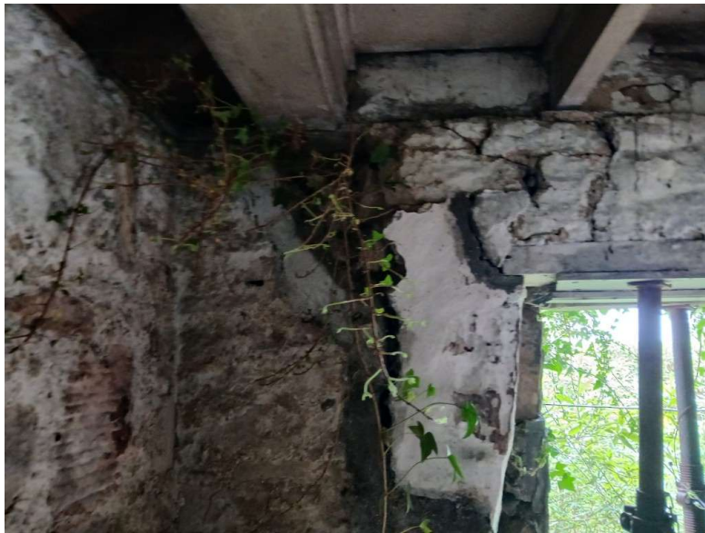
Photograph No.16 – Cracking and dislodged masonry at south-eastern corner and vegetation growing inside building.
