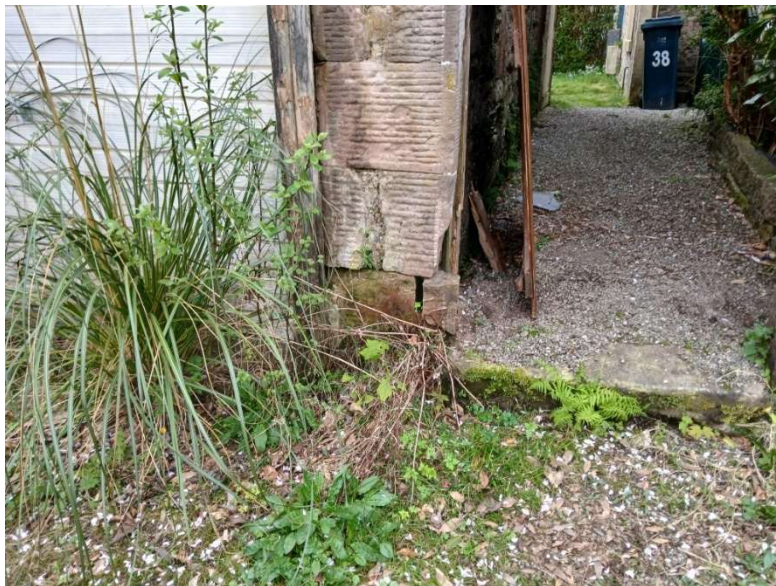
Photograph No.14 – Cracked and dislodged masonry at base course to north-western corner of building.
