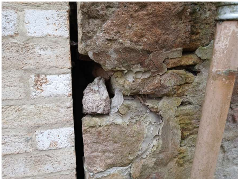
Photograph No.8 – Dislodged masonry below photo 7.
