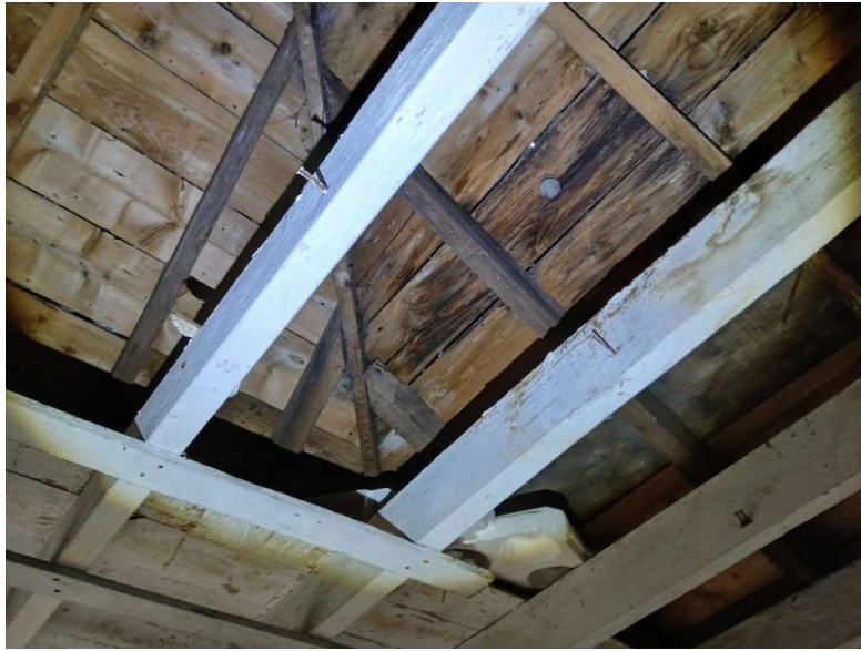
Photograph No.35 – Damp staining to timber elements.
