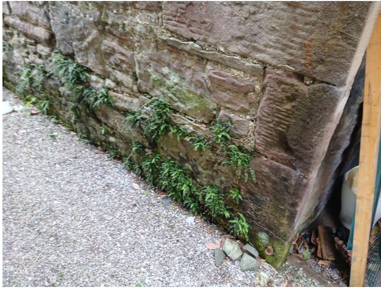
Photograph No.5 – Vegetation growing within bed and perpendicular joints.
